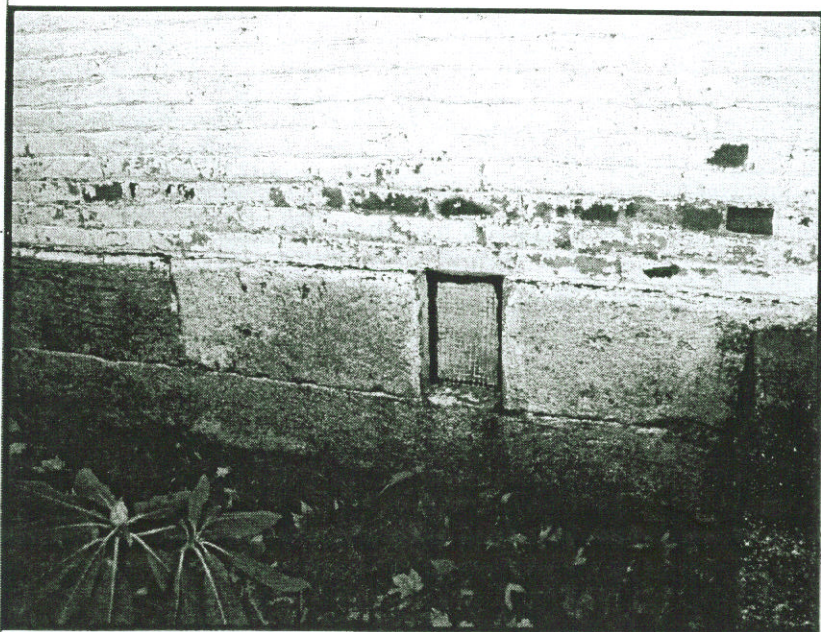
There are several signs of trouble here. Note the algae and staining, indicating that moisture splashing onto the wall is not evaporating. The dark bricks are those on which the painted fronts have spalled off, leaving the inner, softer core of brick exposed. Rising damp is causing the paint to flake off in multiple places—see the clear line of demarcation between damp and dry exhibited by flaking vs. well-adhered paint. Photo courtesy of: Mantero Consulting Group
